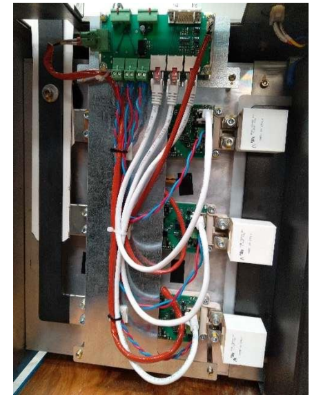
Repaired KACO power stack
